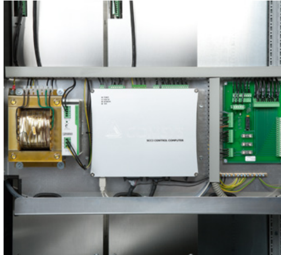
ADF P300 automation panel with the SCC2 control computer.
